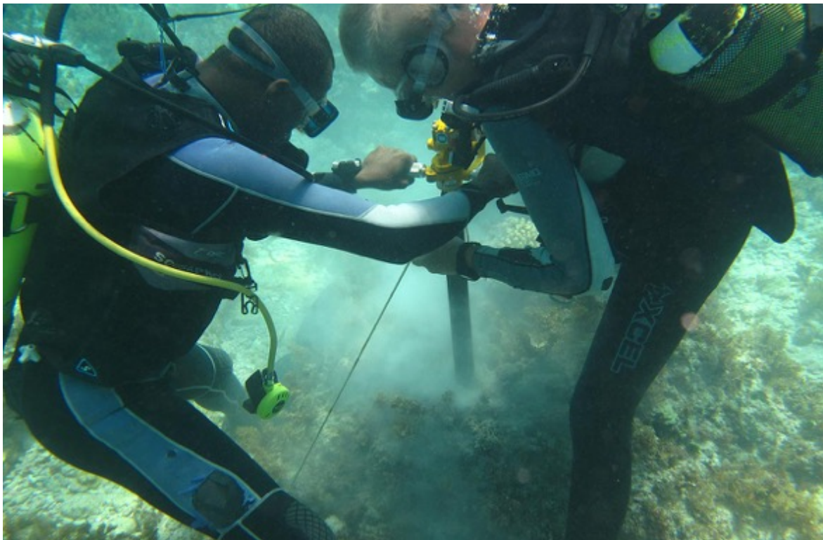
Okala and Chrigel prepare a stable mooring with an underwater hydraulic drill
